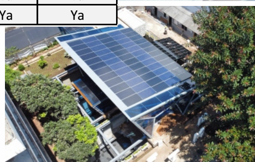
PLTS Teras EBT - FTMD ITB On-Grid, Off-Grid & Hybrid
